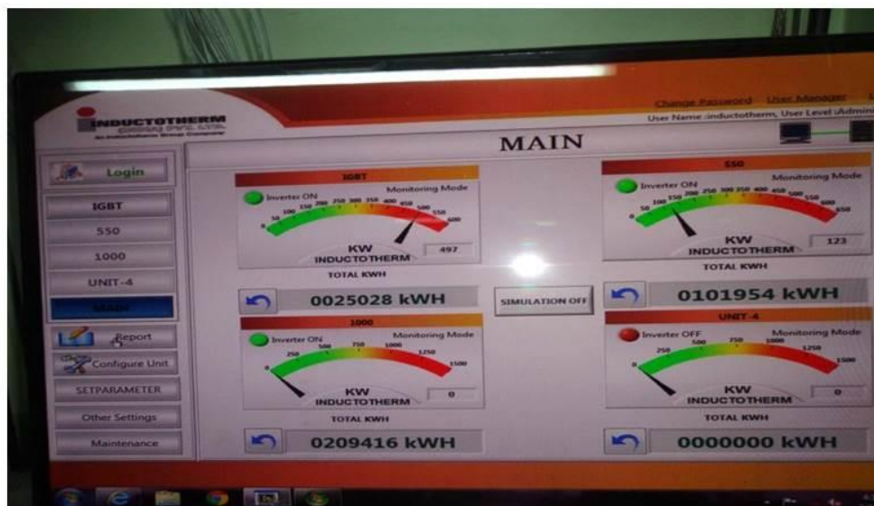
Installation of induction furnace energy monitoring system
